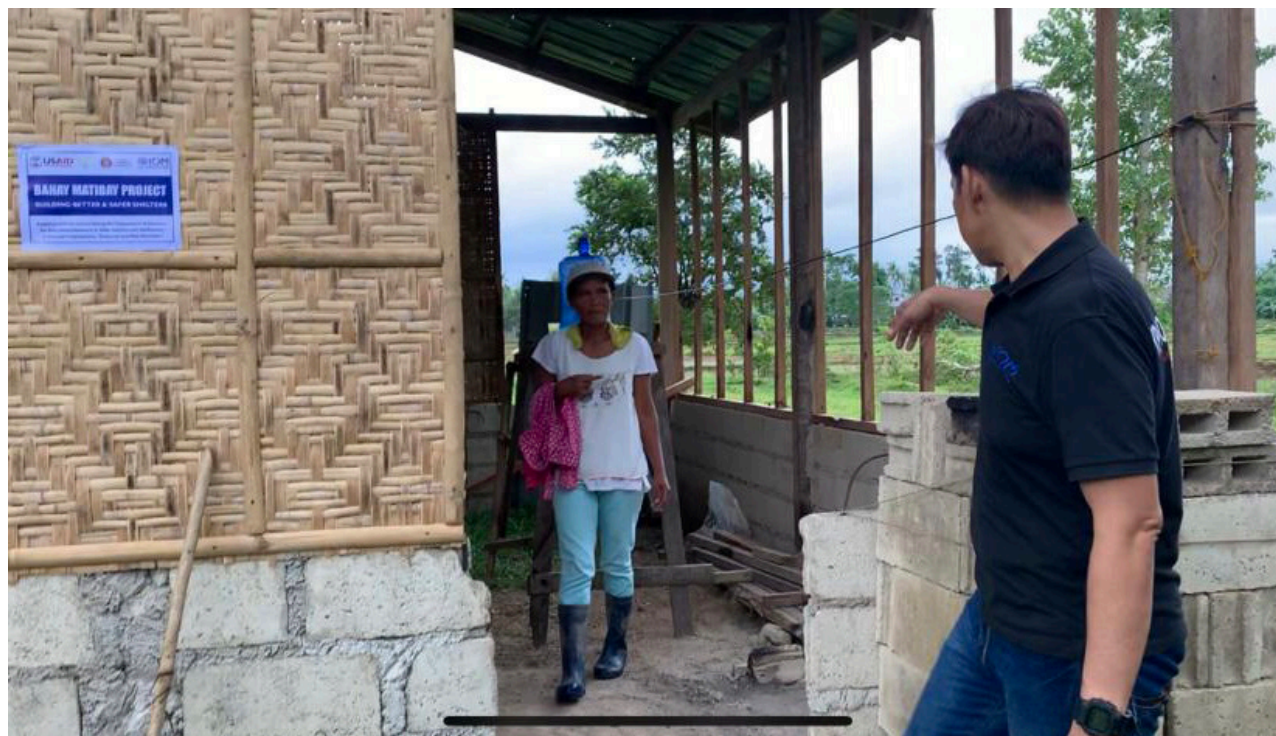
Photo 4: A house under construction in Bohol, constructed in partnership with the Pilipino Senior Resource Center (PSRC). © IOM 2022
